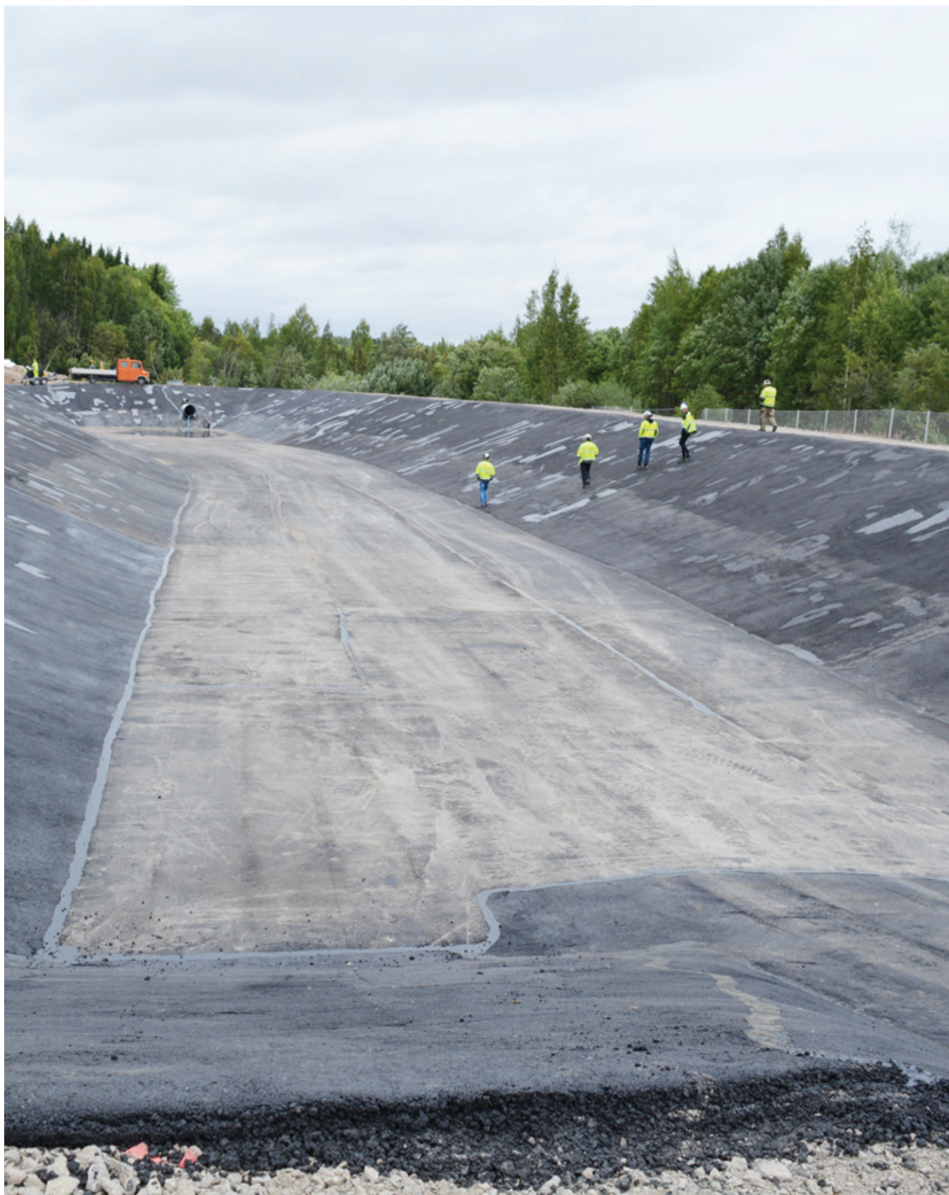
The stormwater detention basin completed in 2018 ensures that the solids present in stormwater runoff, such as fine particles from wood and bark, remain in the basin. This sedimentation basin reduces the nutrient load of the Kymijoki river. The basin is 140 metres long and 30 metres wide, and its depth varies from 3 to 4 metres. The volume of the basin is approximately 5000 cubic metres.
